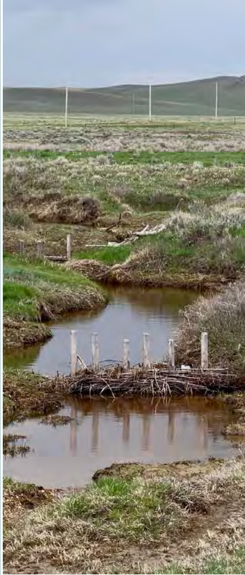
Beaver Dam Analogs (BDAs) installed at Winifred, project site in partnership with the Bureau of Land Management (BLM), Montana Wildlife Federation (MWF), National Wild Turkey Federation (NWF), National Fish and Wildlife Foundation (NFWF), and private landowners. Credit: the Bureau of Land Management
